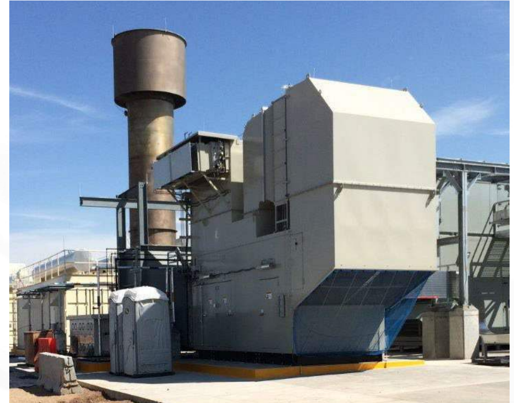
Fuel Tech Data Center SCR System with UDI™ Urea Direct Injection
