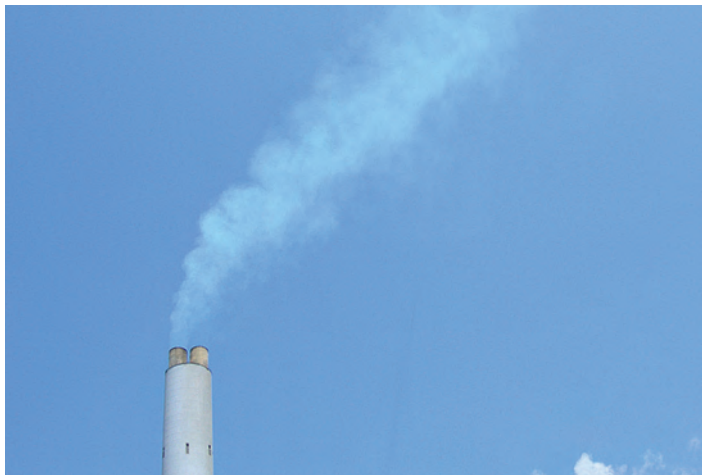
Blue plume clearly visible before TIFI program.
